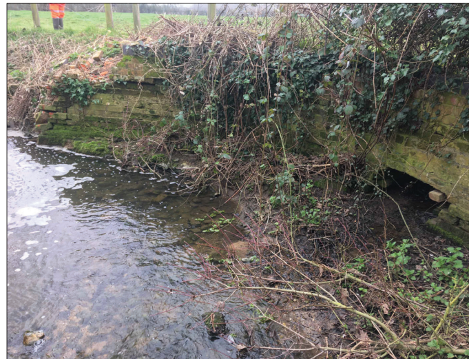
Note 2, Photo 2: Demolish wall and lower field to allow direct flow from culvert to channel during high flows via new, lower level, connecting channel.
